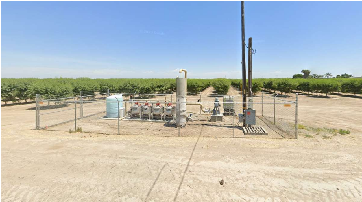
Figure 5-25: Laton Drip Irrigation System
