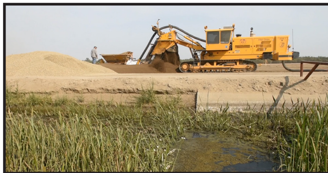
Preparation of site where the perforated pipe is being placed below the surface.
